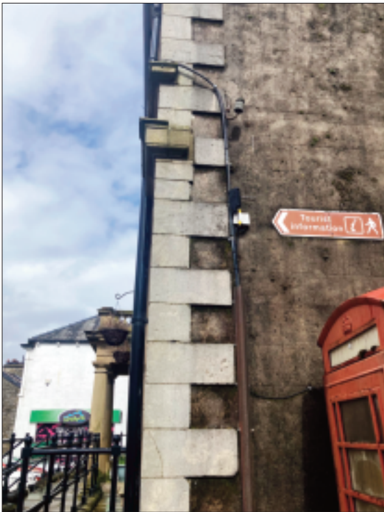
4 Detail of the south west corner of Midland Bank Chambers showing the integration of the new facade (1871-2) with the original building
