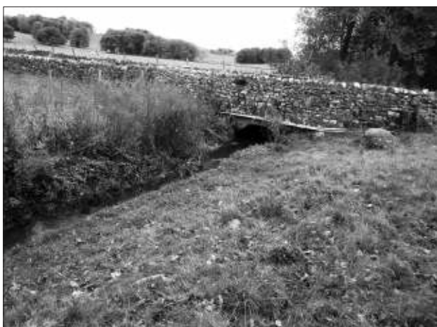
Fig 3 Tarn Dike running under Road
